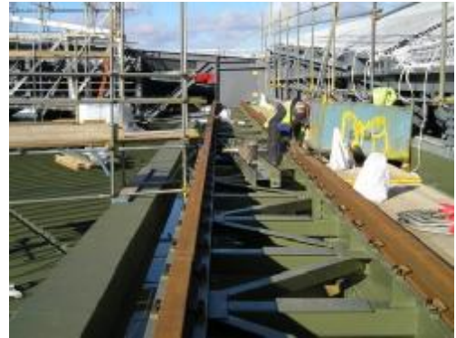
With two rail 'Welding the rails after they had been accurately aligned.'
